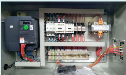
VFD Control Panel
